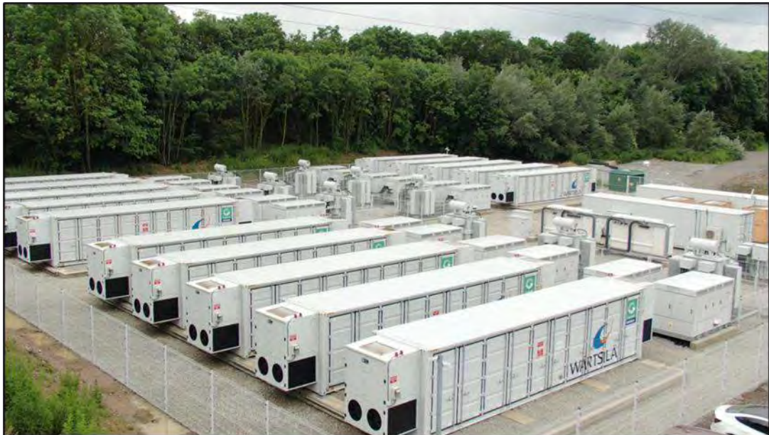
Figure 2-4: Example BESS facility
